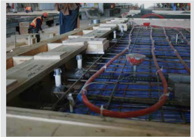
Figure 3. Red cross-linked high-density polyethylene tubes and blue capillary tubes for concrete curing and building climate control are tied to reinforcing steel before placing concrete.
