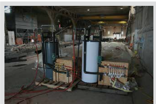
Figure 4. Heating equipment for curing includes two boiler units connected to a circulator pump and manifold for equalizing flow rates through multiple concrete volumes.
